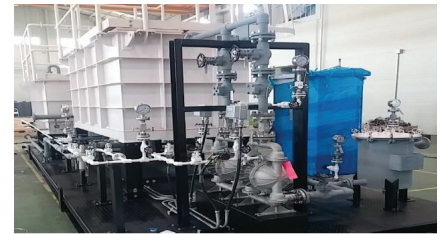
Storm Water Treatment Skid
