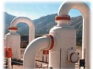
Gas & Water Separation
