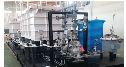
Storm Water Treatment Skid
