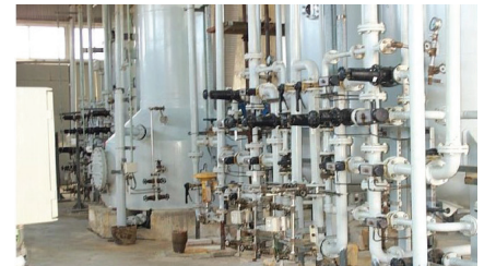
Activated Carbon Filter
