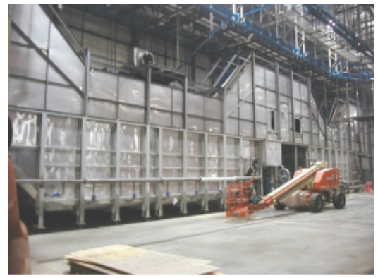
H.M. White Phosphate and E Coat Line Under Construction at an Automotive Plant
