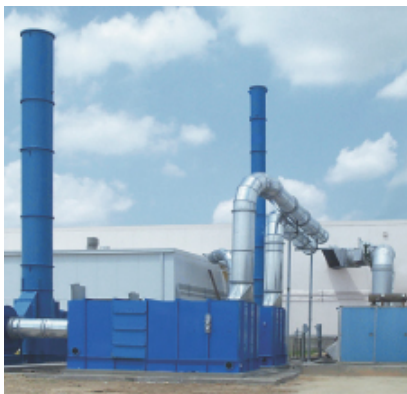
CECO Filters Mist Collector at a Textile Plant
