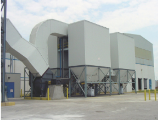
CECO Aire Baghouse at an Aluminum Smelting Facility
